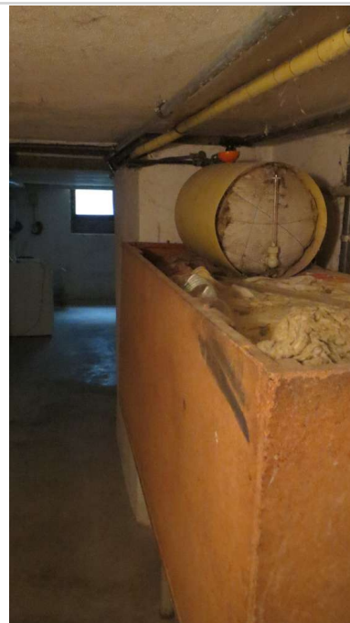
KG WW- Boiler
